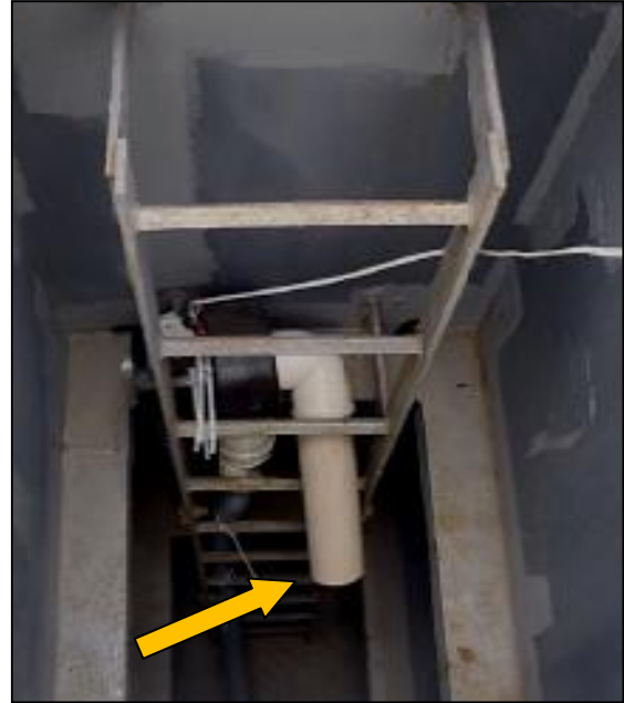
Figure 8: ‘J’ system inlet of suction pipe and recirculation fan in the cargo hold access trunking
