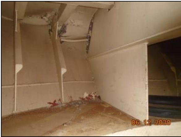
Figure 3: Deformed internal structure in the forecabin store
