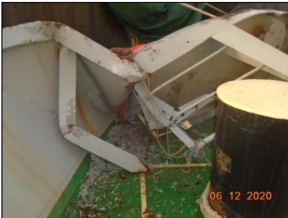
Figure 4: The damaged bulwark on the bow of Atlantic North
