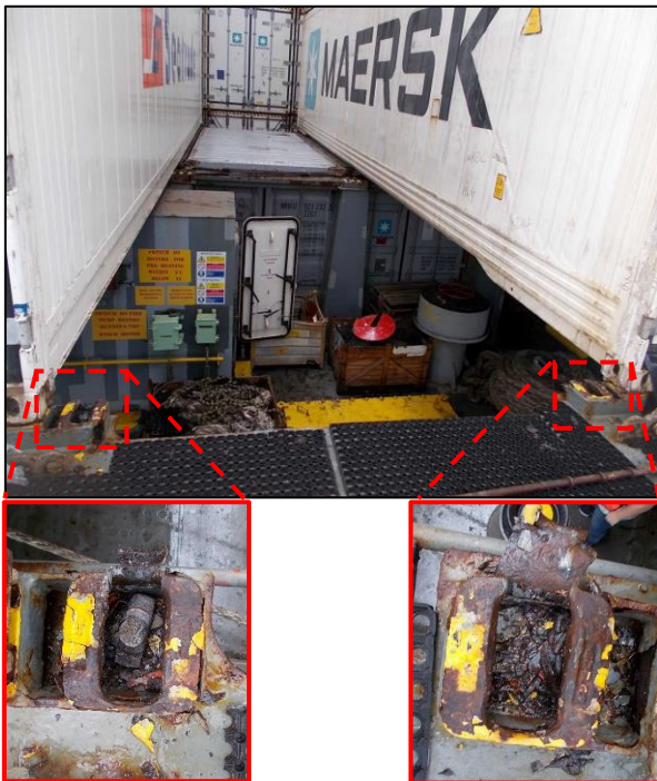
Figure 5: Damaged deck container sockets
