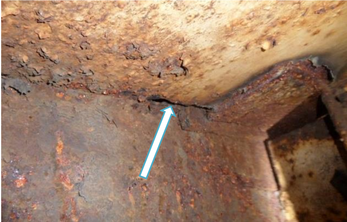
Photograph 6. Cracks in the upper part of the air conditioning ventilation trunk on welded joints of metal sheets in the ventilation casing of ship starboard side cargo hold.
