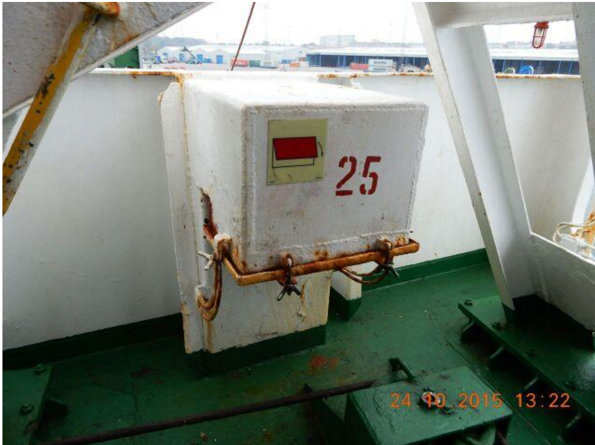
Photograph 5. Air conditioning inlet in ship superstructure on boat deck on starboard side.
