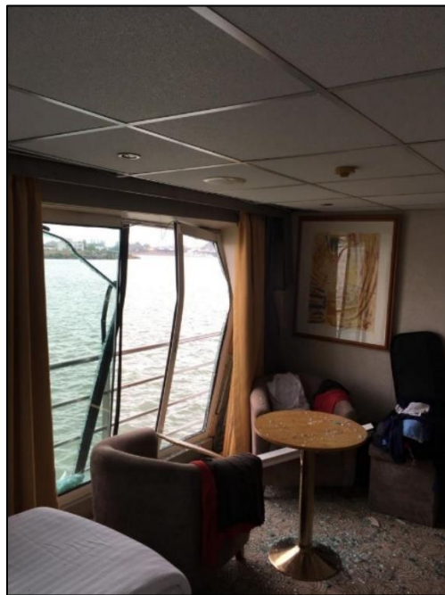
Figure 5.7 – Damages to Cabins
