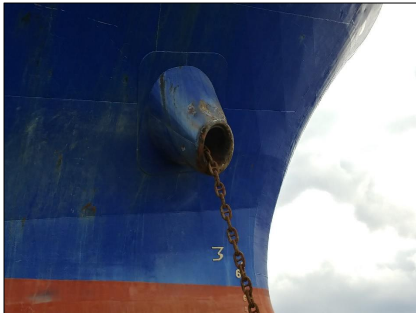
Figure 5.10 – Scratches on coating
