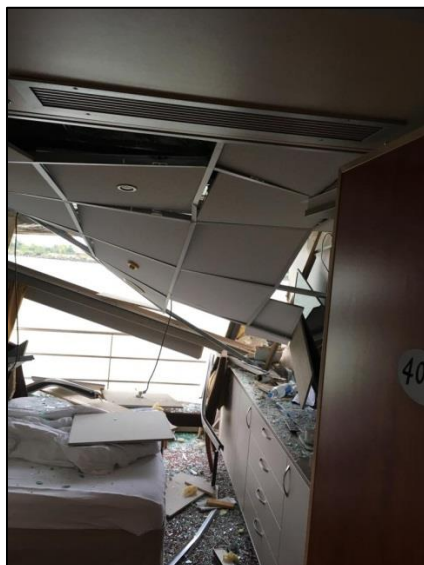
Figure 5.3 – Damages to Cabins
