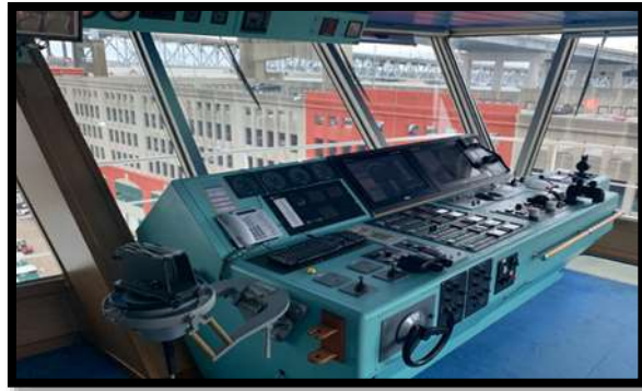
Figure 5.5: starboard bridge wing, RADAR: SA 164632051 WARTSILA COMPASS SAFE DISTANCE Sam electronic S: AZ3073G240. ECDIS Chart: MX509225, MAIN AND STBS SIDE, CONN FULL BRIDGE: MULTIPILOT PLATINUM \ RADAR SYTEM WITH AUTOMATIC RADAR PLOTTING AID MEETS THE REQUERIMENTS IMO A.694 (17) AND A.278 (VII) S:IEC 62388,IEC 60945 , IEC 62288 .
