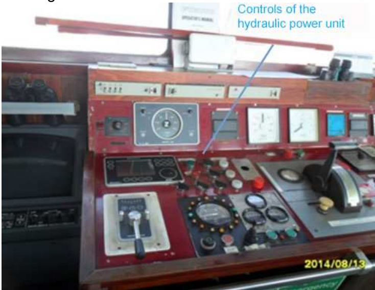
Port side control panel, looking towards the bow of the vessel.
