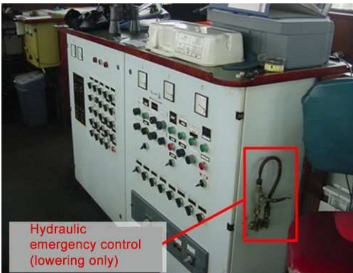
View of the electrical panel from the port side looking aft of the wheelhouse.
