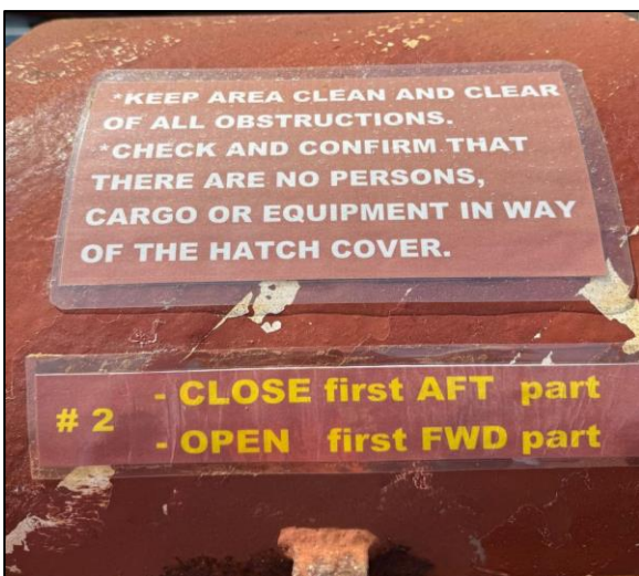
Figure 5: The instruction posted on the hydraulic control station
