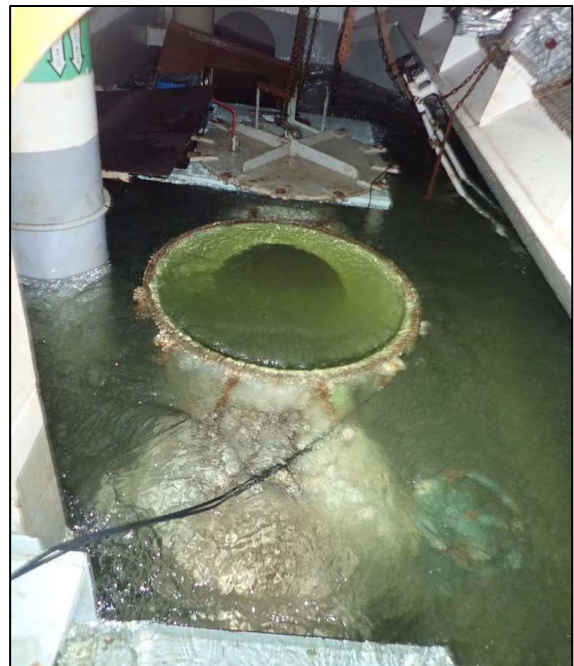
Figure 3: The open strainer housing (photograph taken after the sea chest valve was shut)
