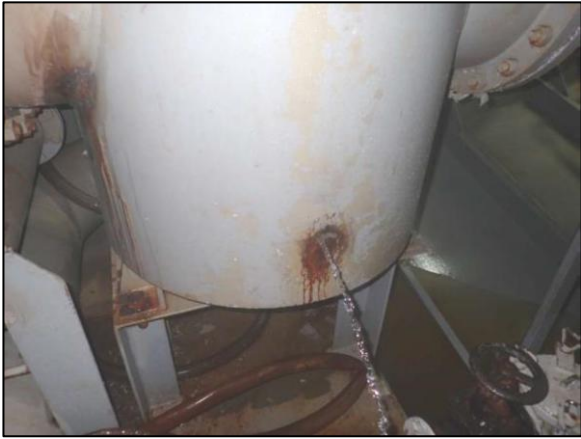
Figure 2: The leaking strainer housing
