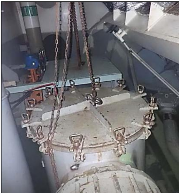
Figure 7: Port side sea chest, showing the cover secured in place
