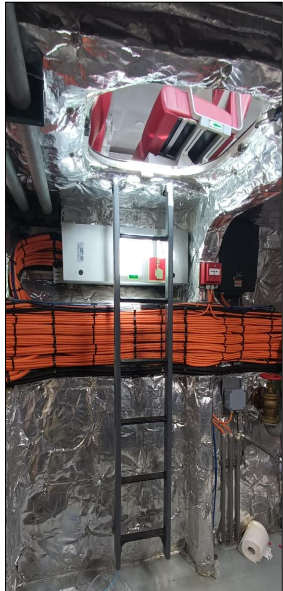
Figure 4: Port switchboard escape ladder and open escape hatch cover
