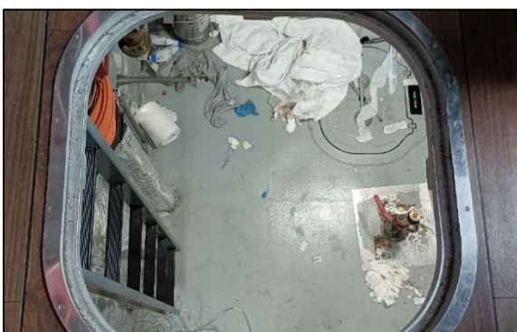
Figure 3: Port side switchboard room from the passenger hall
